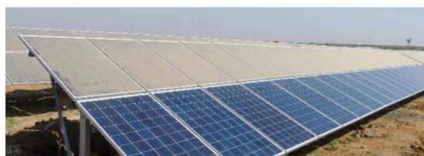
UNTREATED TOP HALF OF SOLAR PANEL
